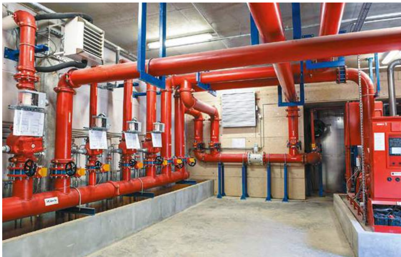
Sprinkler system at Sferaco.
