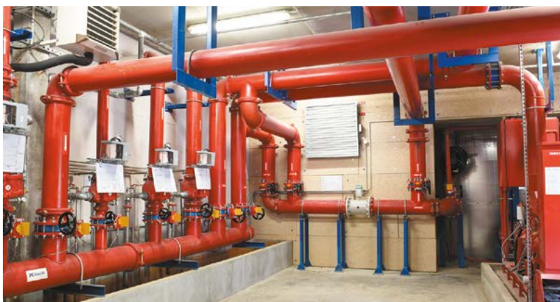
Sprinkler system at Sferaco.
