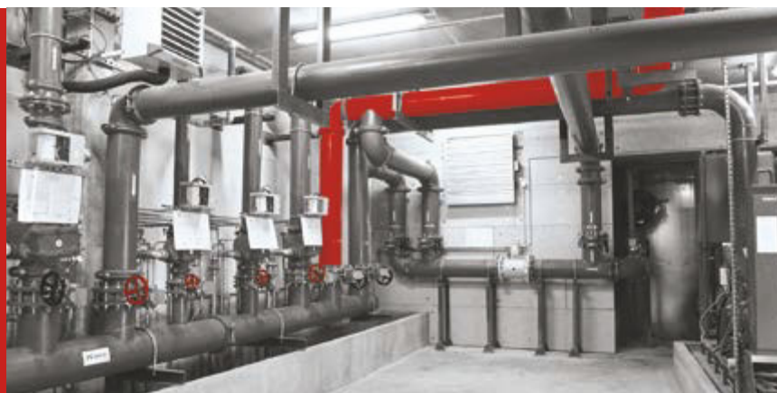
Sprinkler system at Sferaco
