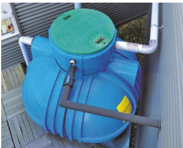
Globus rainwater recovery system at Jetly
