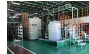
Water recycling equipment
