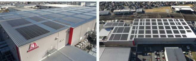
Rooftop solar power generation system installed at Takasaki Morinaga Co., Ltd.
