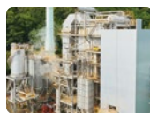
2007 Taiho Paper Introduction of a biomass boiler
