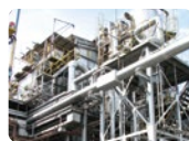
1983 Eco Paper JP Introduction of a biomass boiler
