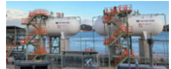
Ammonia supply facilities
