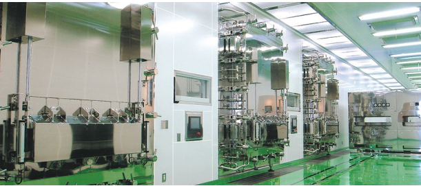
Freeze dryers and automatic guided vehicles (AGV)
