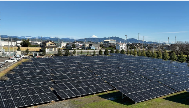
Solar Power Generation (Fujieda Site)
