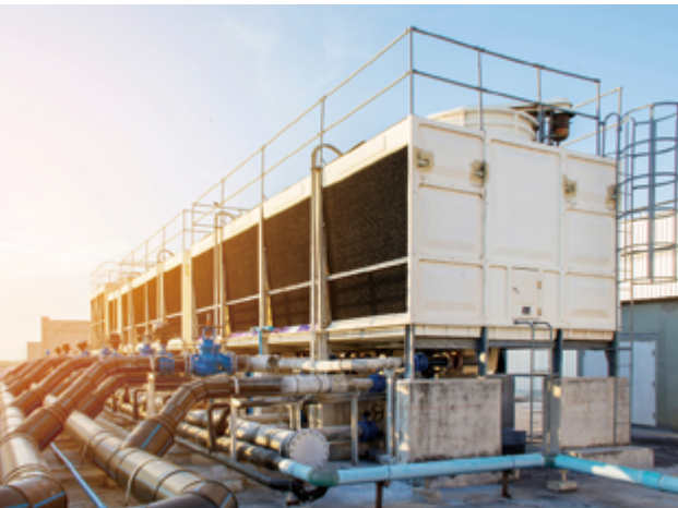
Image of cooling tower
