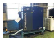
New compressor in the ironworking plant
