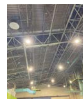
Interior LED lighting
